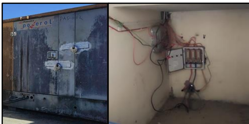
Energy conservation facilities observed in the Campus
